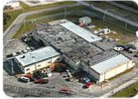
Cram Roofing replaced the roof atop the Communication Building at NASA's Kennedy Space Center in Cape Canaveral, Fla. The job totaled approximately 348 squares. (Photos courtesy of Cram Roofing.)
